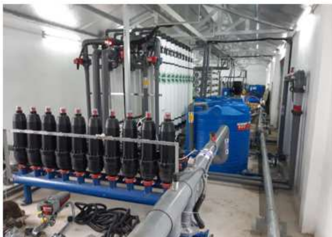
Water recycling system
